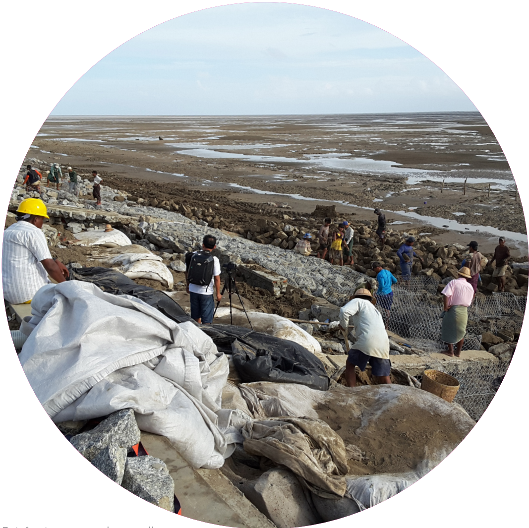
Reinforcing a coastal sea wall in Khin Dan village, Mon State, Myanmar.
