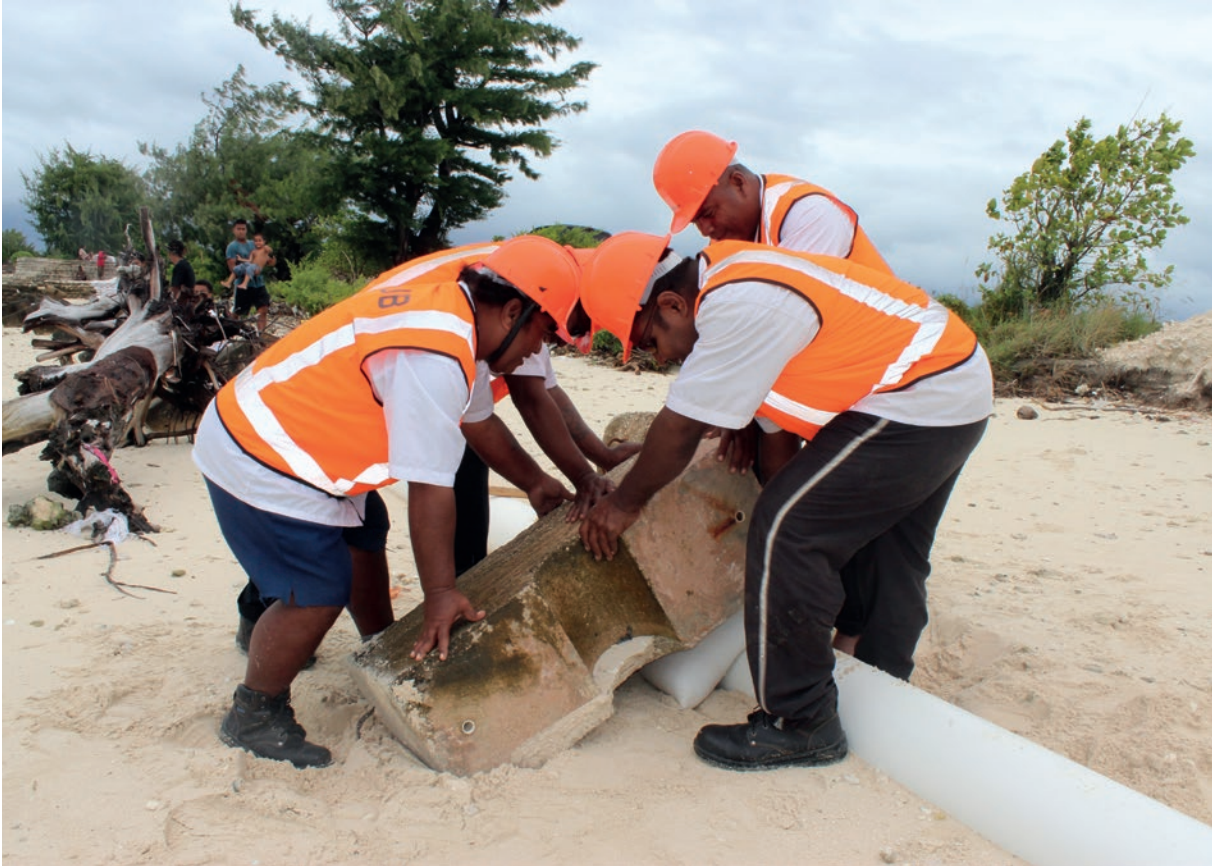
Workers from the Public Utilities Board putting pressure onto water pipes to ensure they are not moved or damaged during high tides, Ambo village, Kiribati, February 2013.
